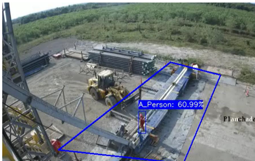
Figure 3—Worker exposed to moving mechanisms - Image of video analytics model for detection people, captured by the system.
